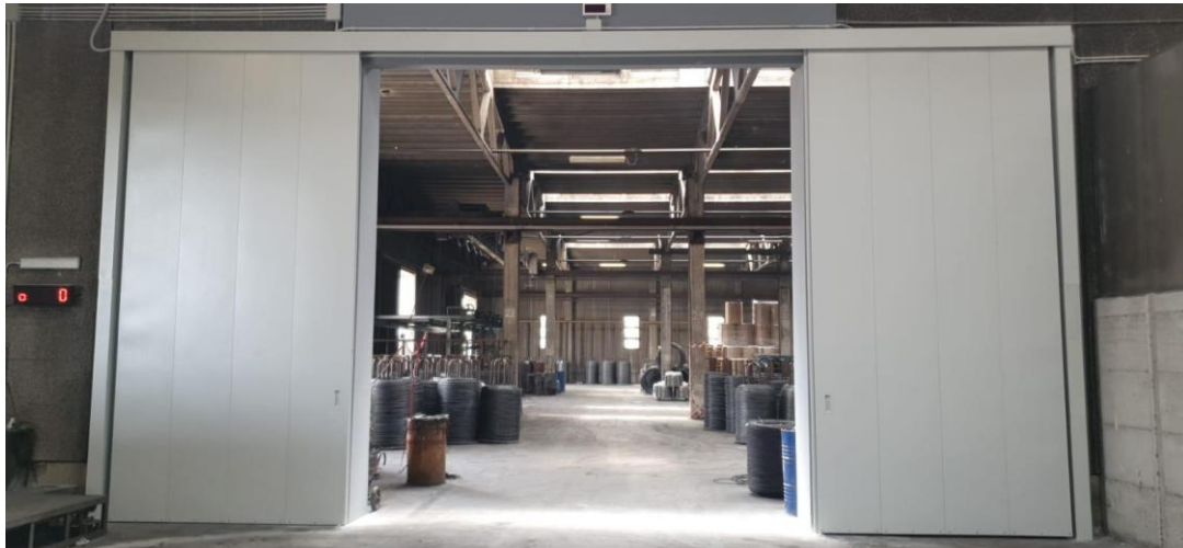
Figure 2: Sliding fire door
