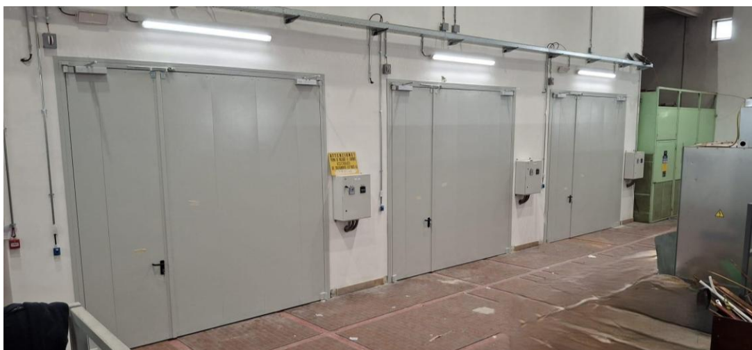
Figure 3: Large-Dimension hinged fire doors
